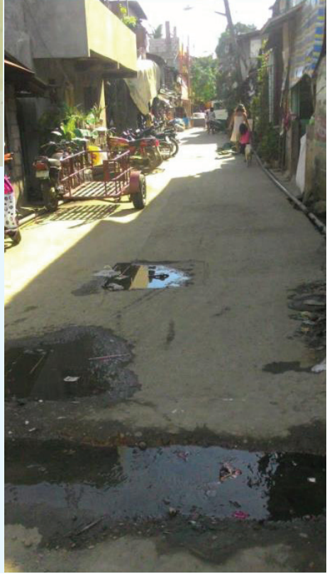
Potholes in the paved roads that traverses the settlement
