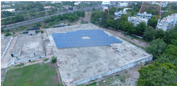
The 145 kW Solar PV system installed at one of Rajkot's water treatment plant, as part of its Urban-LEDS response in phase 1
